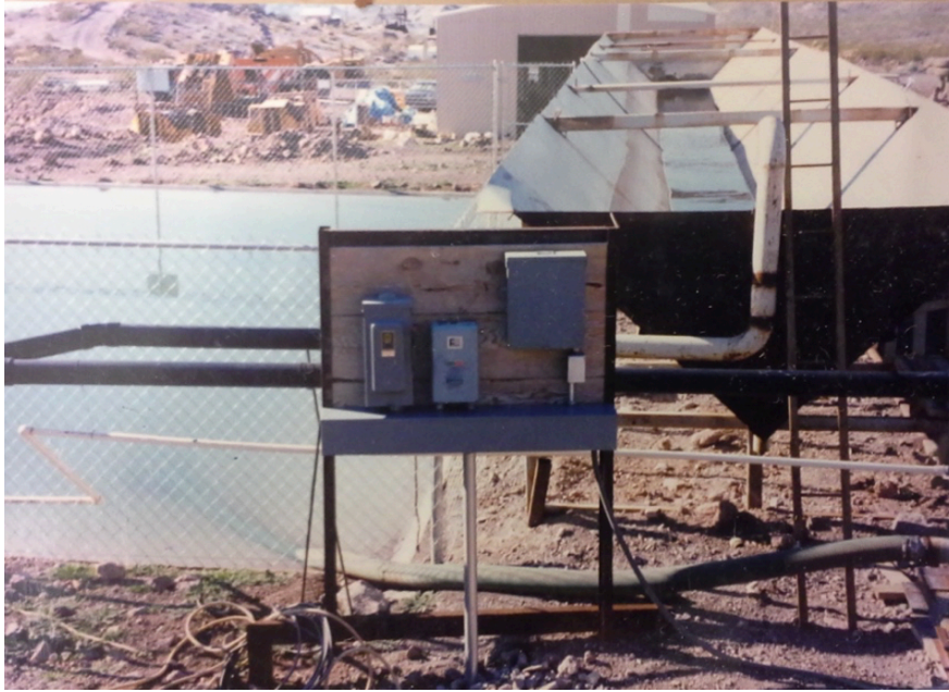
Figure 1.5: PLS Distributer Channel and Holding Pond [3]
